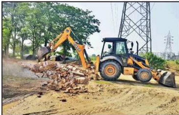
A team from Gmada removed the squatters living in four to five illegal structures which were obstructing the construction of the road
