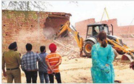
The enforcement staff of GMADA pulls down an illegal structure in Mohali on Saturday. A TRIBUNE PHOTOGRAPH
