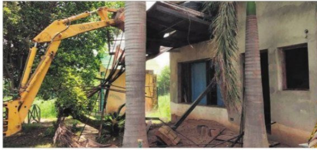
GMADA officials raze an illegal structure with a JCB machine in Mohali district. TRIBUNE PHOTO
